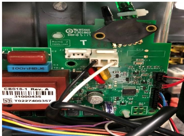
Figure 19. Main Board with Attached Harnesses
